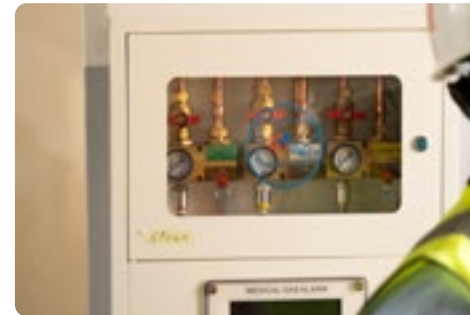
Medical gas installation at the South Ward of the MCOE. Photo by Chiara Herold / PIH
